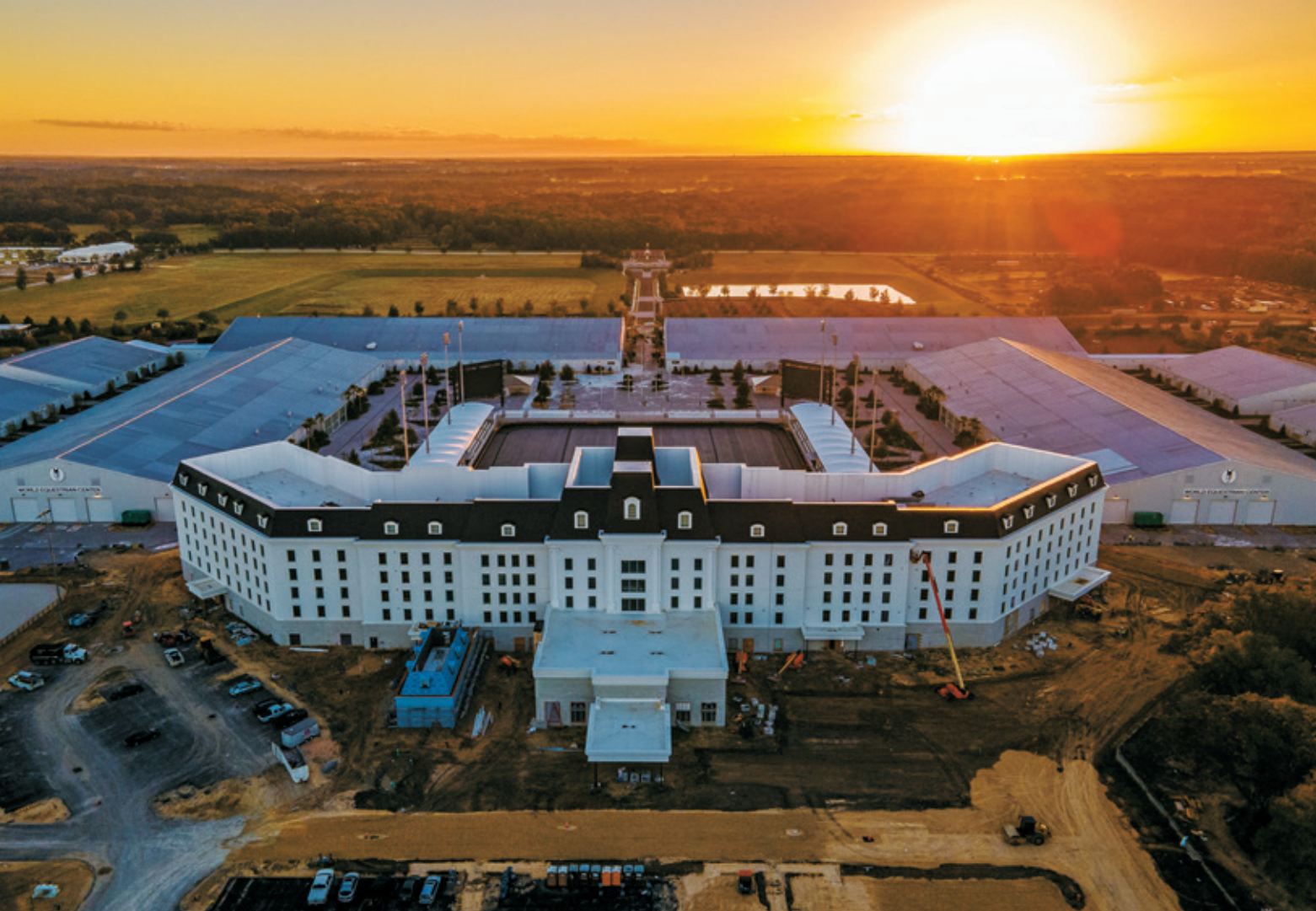
World Equestrian Center, seen here while under construction, continues to drive interest in Ocala area farms
